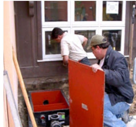
Michael Petty (front) and Tony Bernardasci of A&R Plumbing install a grease trap at the Youth Center.
