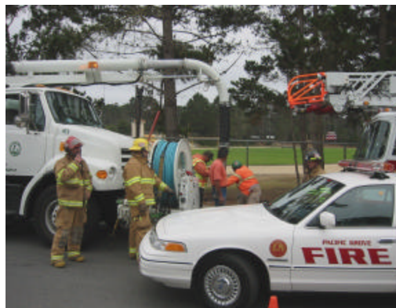
Fire and Sewer Crews work together to stop effluent escaping from private property line rupture.
