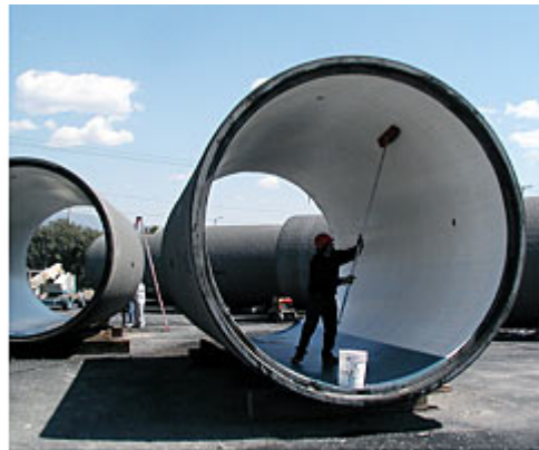
Preparation of pipe for installation in the new Northeast Interceptor Sewer. Photo courtesy of the City of Los Angeles
