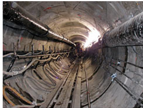
Tunneling for installation of the new East Central Interceptor Sewer. Photo courtesy of the City of Los Angeles
